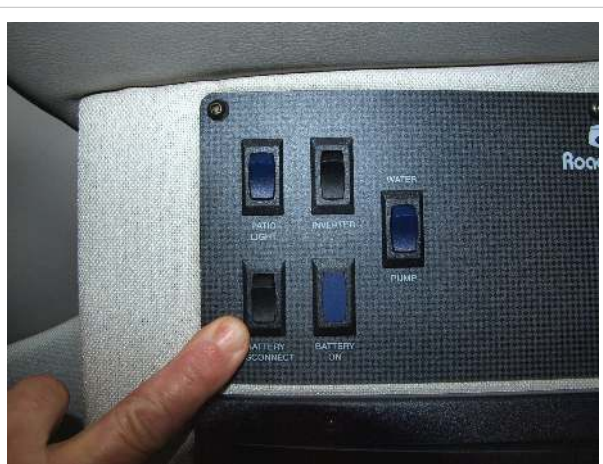
Battery disconnect switch
