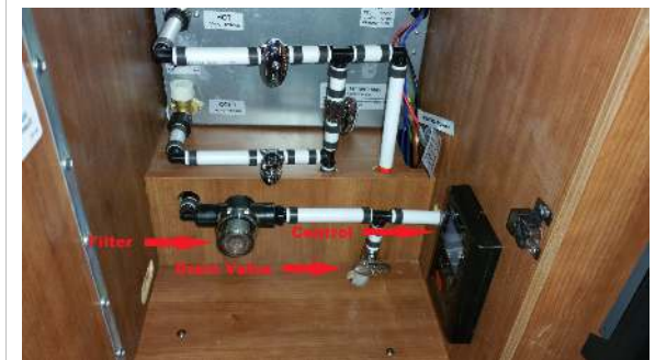
Tankless water heater drains
