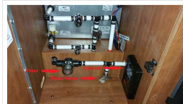
Water heater thermostat, filter and drain valves
