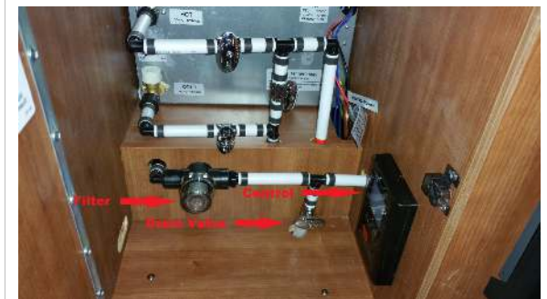
Tankless water heater drains
