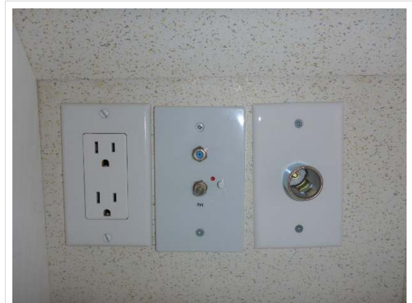
TV Antenna and Cable connections.
