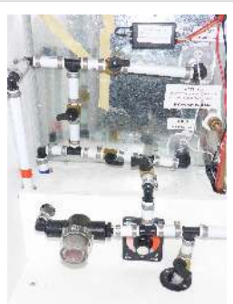
Tankless water heater inside cabinet - all valves are in normal operating position
